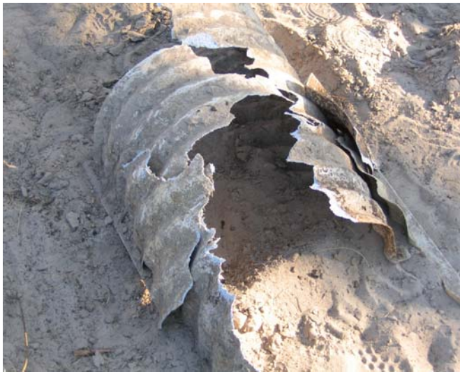
Septic systems can become damaged, allowing hazardous wastewater to leak.
