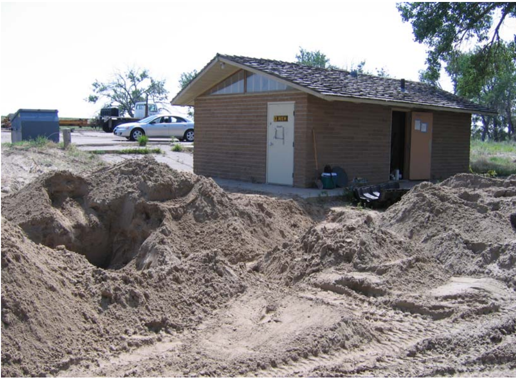
Proper maintenance can extend the life of a septic system, preventing the inconvenience and cost of installing a new system (as seen here), as well as preventing pathogenic contamination.
