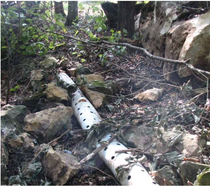
Failing on-site wastewater systems threaten groundwater resources.
