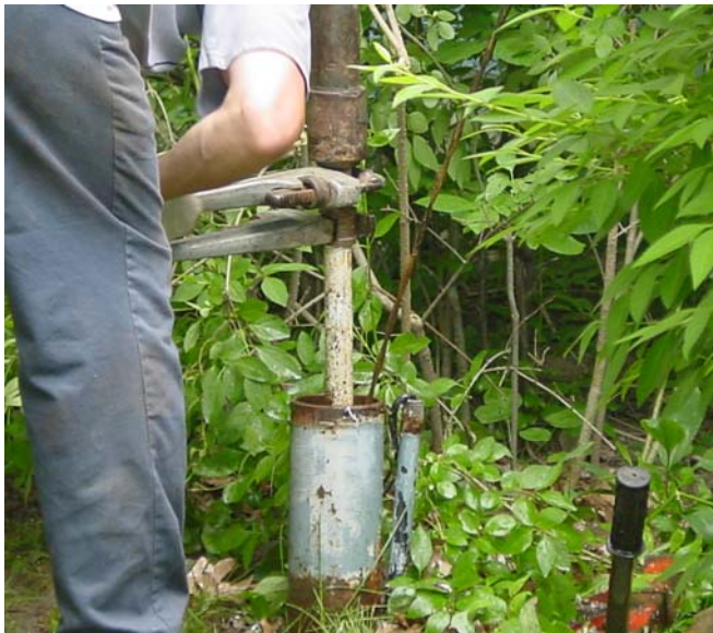
This abandoned well was properly decommissioned as part of the Greater Lansing Area's wellhead protection activities.
