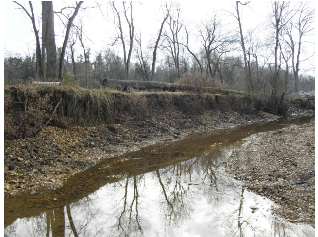
An eroding streambank and site of upcoming restoration work
